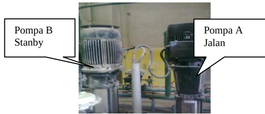
Gambar 4.2 Pompa Air Cooling Tower
